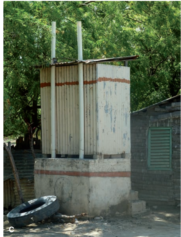
FIGURE 7-3 (Continued) B. An Ethiopian pit latrine, which offers no mitigation for flies and is situated in proximity to the water table below. Heavy rains will lead to contamination of the water supply with fecal pathogens. (Courtesy of Richard P. Usatine, MD.) C. An elevated, ventilated improved pit latrine can protect the water table and reduce flies. Air circulates down the squat hole, into the pit and up through the pipe. To ensure unhindered flow of air, the top of the vent pipe must be 0.5 meters above the top of the shelter. The latrine interior is kept dark so the main light source in the pit comes from the vent pipe. Flies are attracted to the light, but the pipe has a fly-proof screen at the top, so they cannot escape and eventually die. 5 Many countries consider the ventilated improved pit latrine to be the minimum standard for improved sanitation. (Courtesy of Jason Rosenfeld, MPH.)
